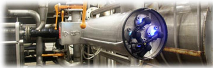
Drinking Water Treatment (UV/H 2 O 2 system)
