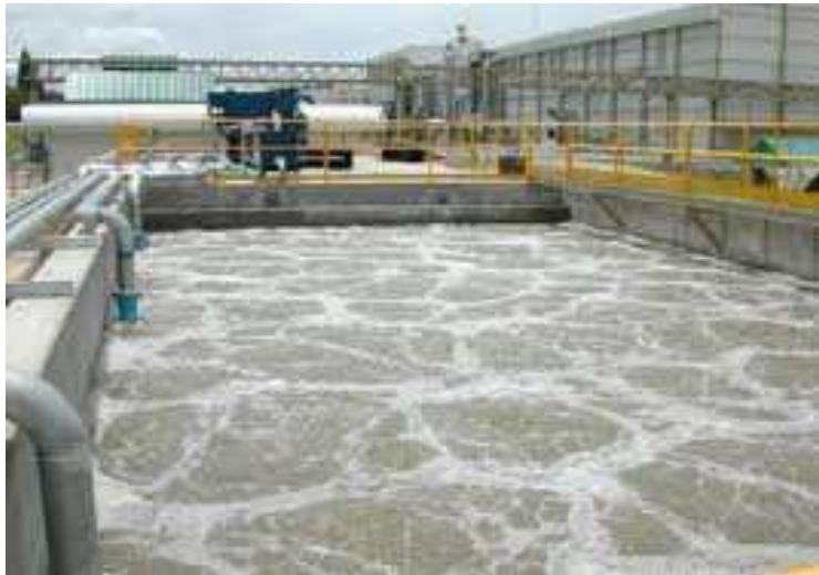
Biological wastewater treatment
