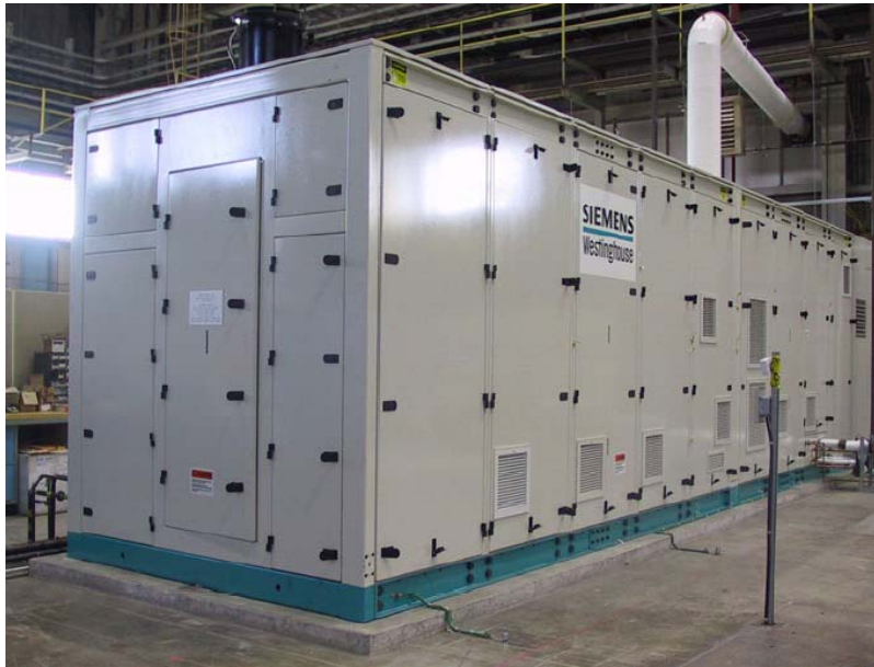
Figure 7-28 Siemens Westinghouse 250 kW Tubular SOFC Installation (31)
