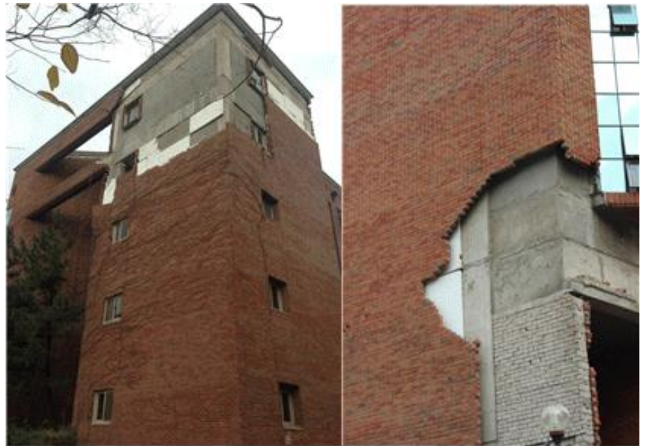
Falling of masonry wall
