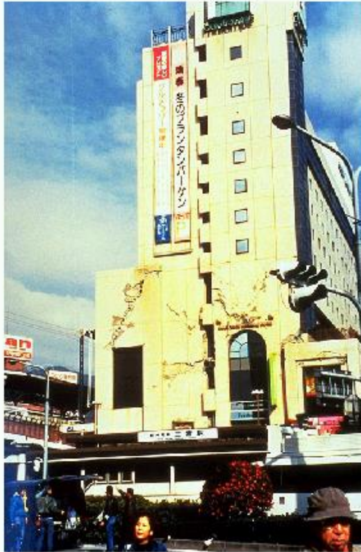
Severe damage to relatively modern hotel structure in downtown Kobe. While the majority of partial or complete collapses appear to be older, reinforced-concrete buildings (pre-1975), severe structural damage was also observed for buildings of steel or composite construction.
