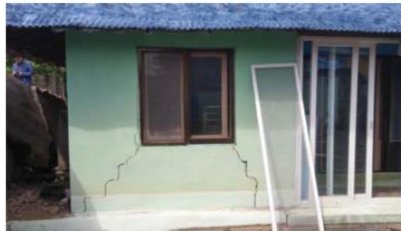
Typical corner cracking at opening
