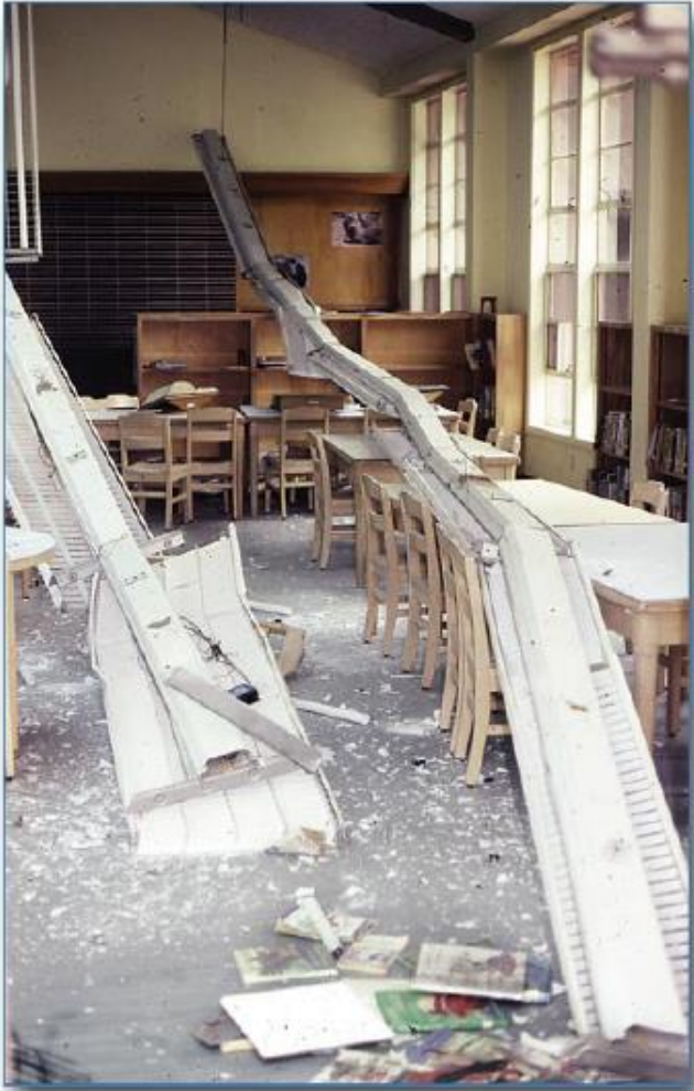
Falling of ceiling
