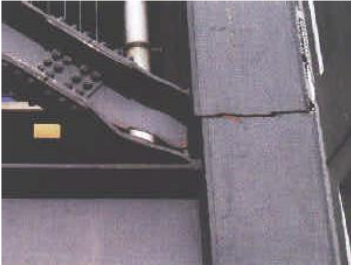
Fracture of steel tube column with thick plates
