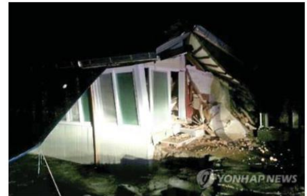
Failure in an already poor (non-engineered) construction
