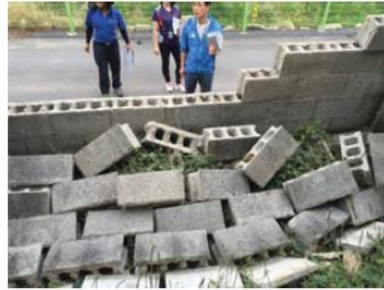
Unreinforced block wall fallen down
