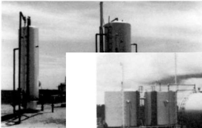
Figure 1-30. An onshore lease facility featuring a horizontal two-phase separator.
