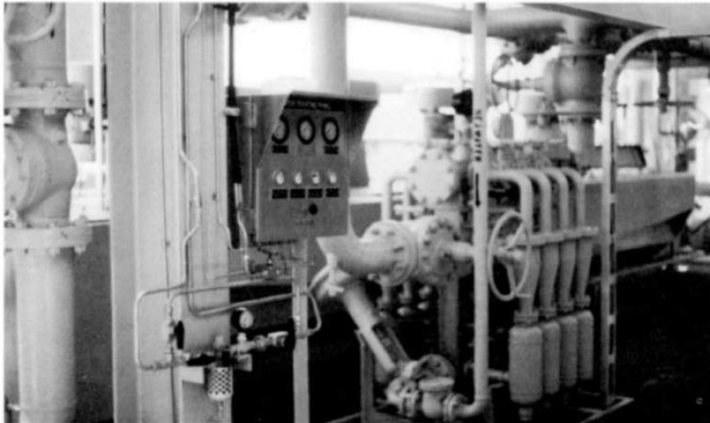
Figure 1-13. Hydrocyclone desanders used to separate sand from produced water prior to treating the water.
