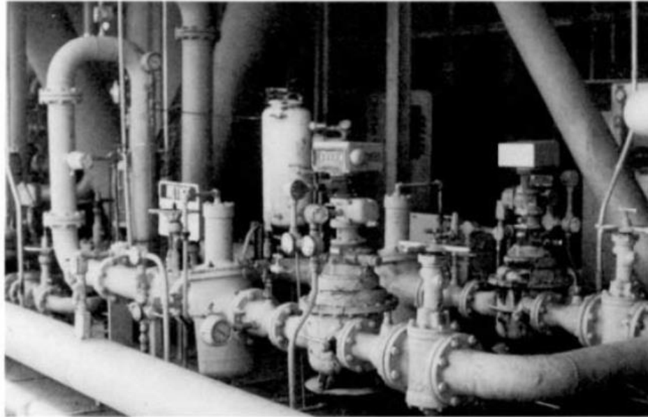
Figure 1-10. A LACT unit for custody transfer of oil. In the vertical loop on the left are BS&W probe and a sampler unit. The flow comes through a strainer with a gas eliminator on top before passing through the meter. The meter contains devices for making temperature and gravity corrections, for driving the sampler, and for integrating the meter output with that of a meter prover (not shown).
