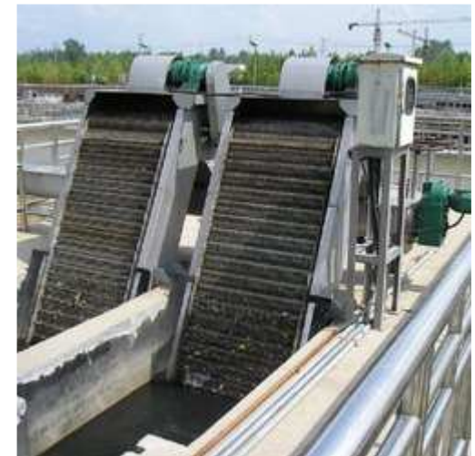
Mechanically-cleaned bar screen
