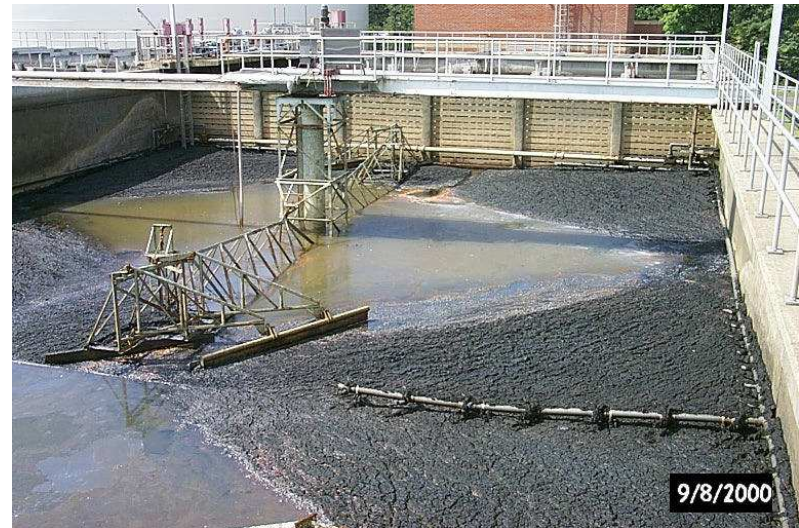
Sludge in the sedimentation basin
