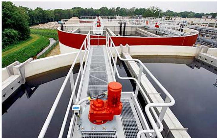
WWTP in Epe, the Netherlands (2010~)
