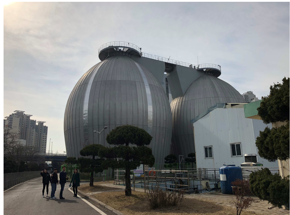
Biogas storage tank
