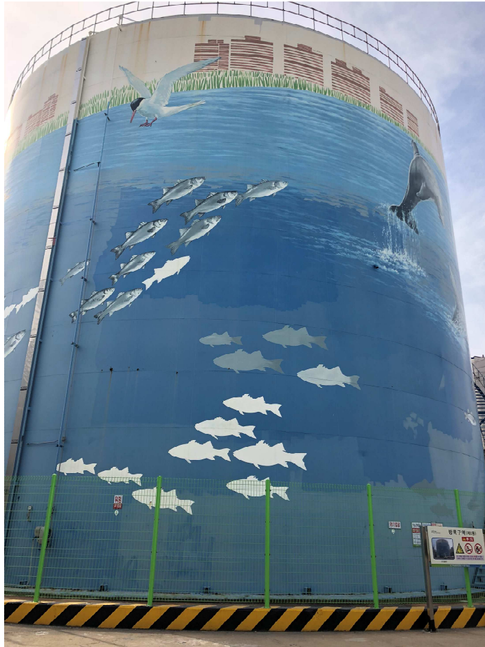
Anaerobic digestion tank
