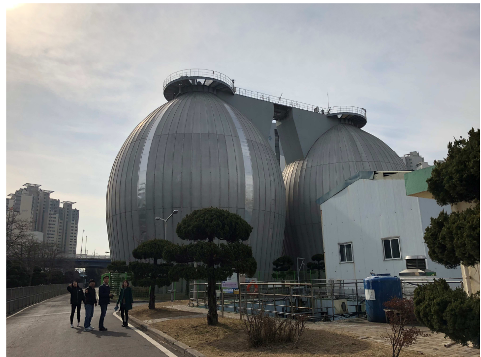
Biogas storage tank
