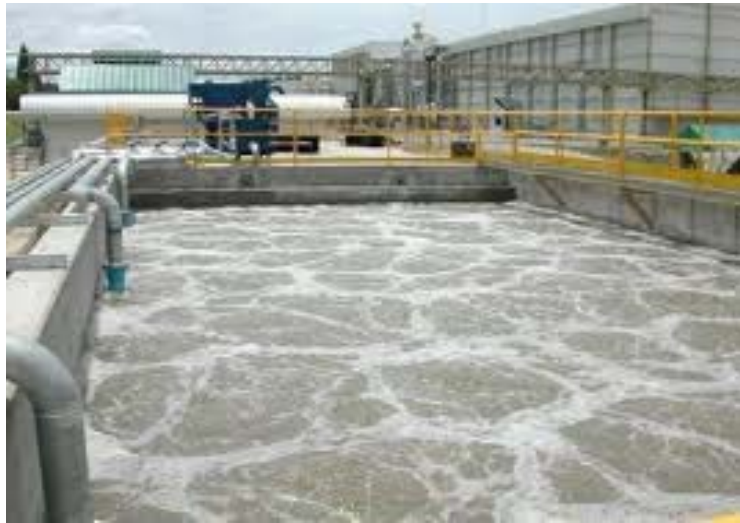
Biological wastewater treatment
