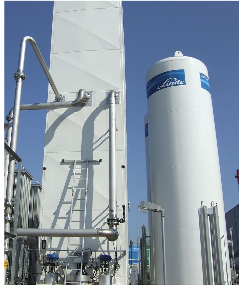
Distillation column in a cryogenic Air separation plant
