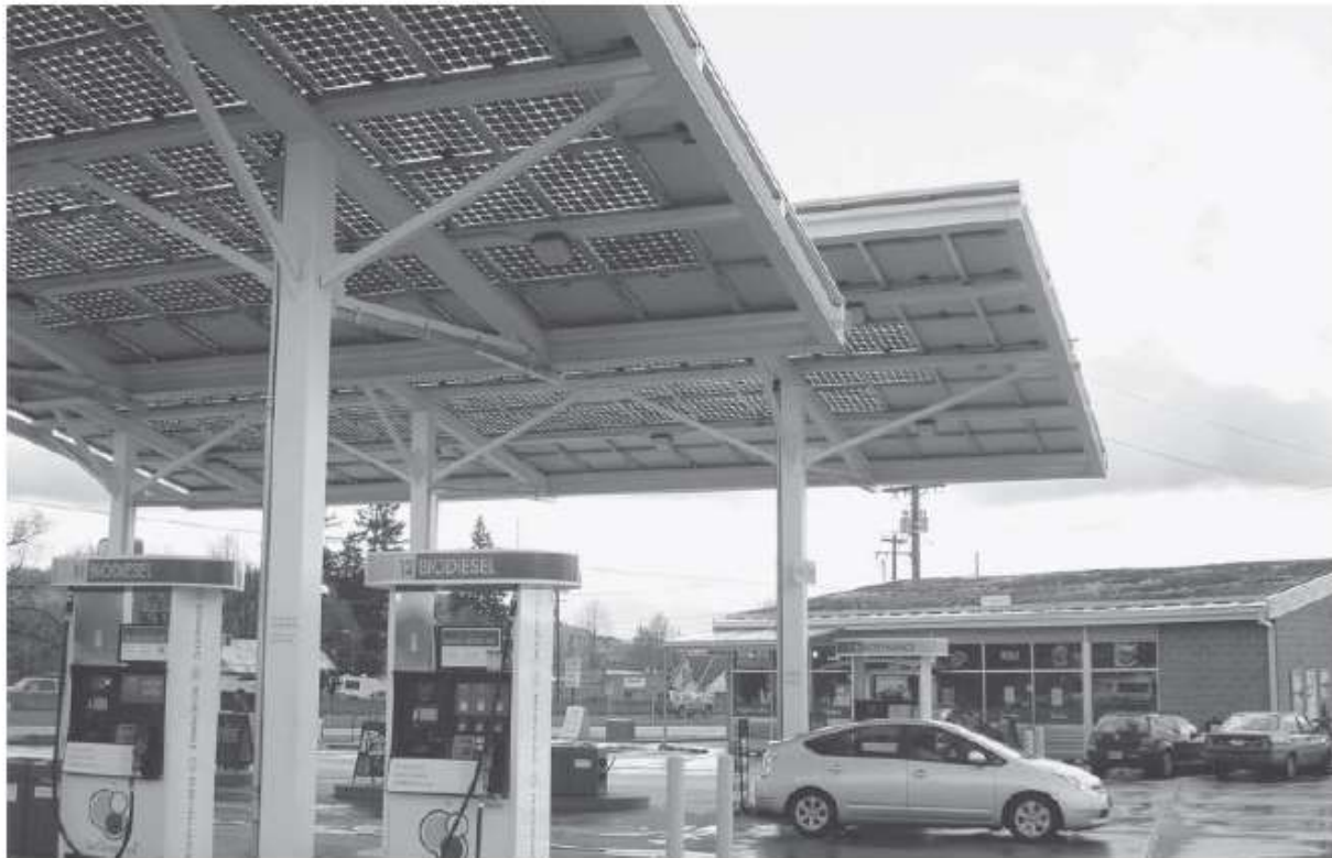
Fig. 2.8 "Building"-integrated photovoltaics (BIPV) provide shelter, shading, and power for a fueling station/convenience store in Eugene, Oregon. Note the green roof on the store and the biofuel pumps. (Photo by Nathan Majeski.)
