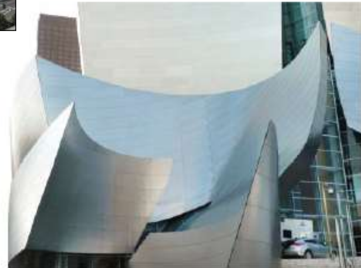
Fig. 3.20 After construction, modifications were made to the highly polished stainless steel exterior of the Walt Disney Concert Hall in Los Angeles, California (by Frank Gehry), to reduce reflections impacting the neighboring condominiums; surfaces now have a matte finish. (© Karen Tse; used with permission.)
