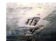
Corrosion of exposed rebar
